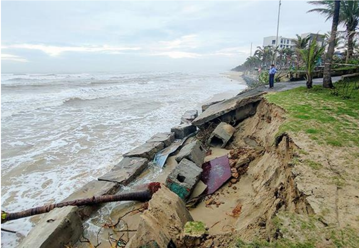
The coast of the Ngu Hanh Son district underwent severe erosion, starting in December 2020.
