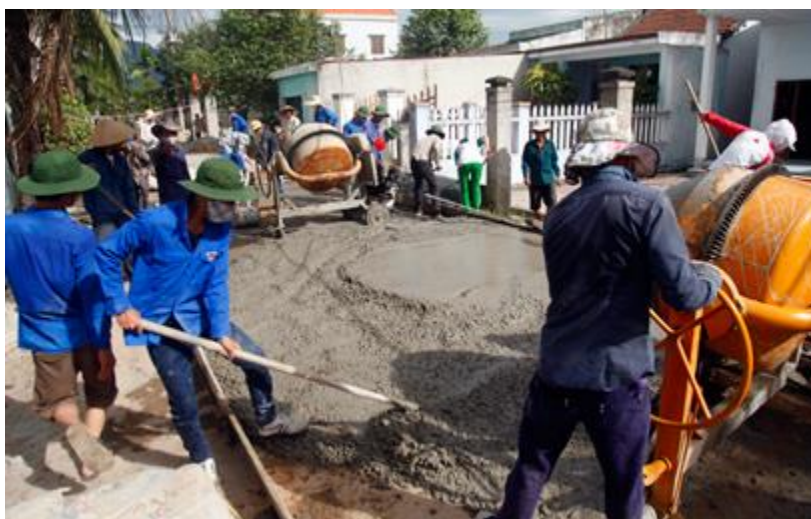
DTU students help local residents build a road
