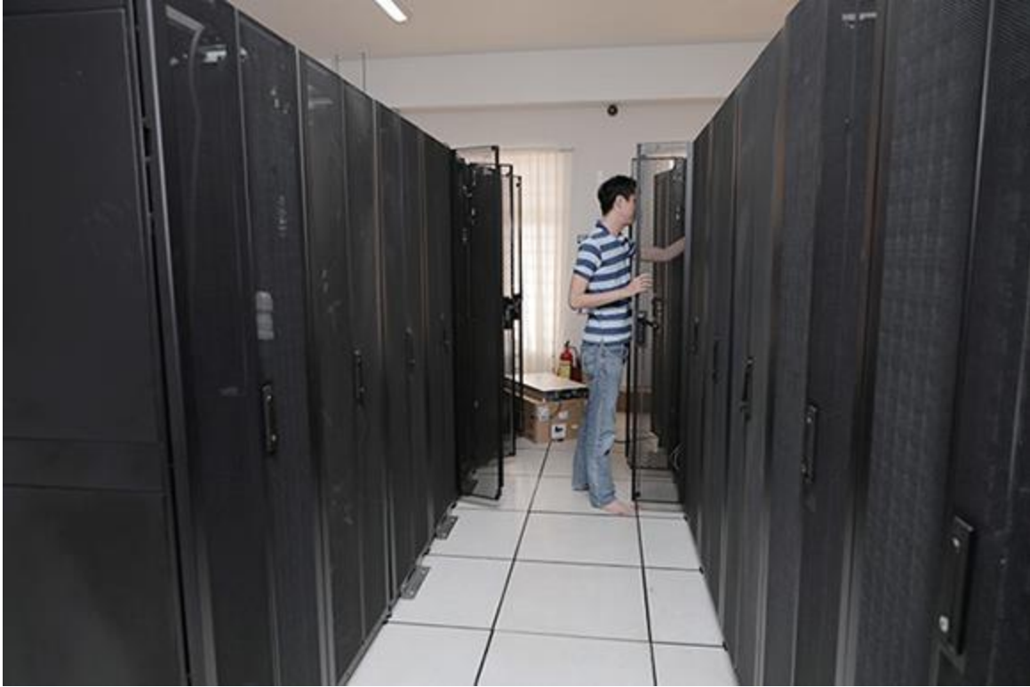
The Data Center support
