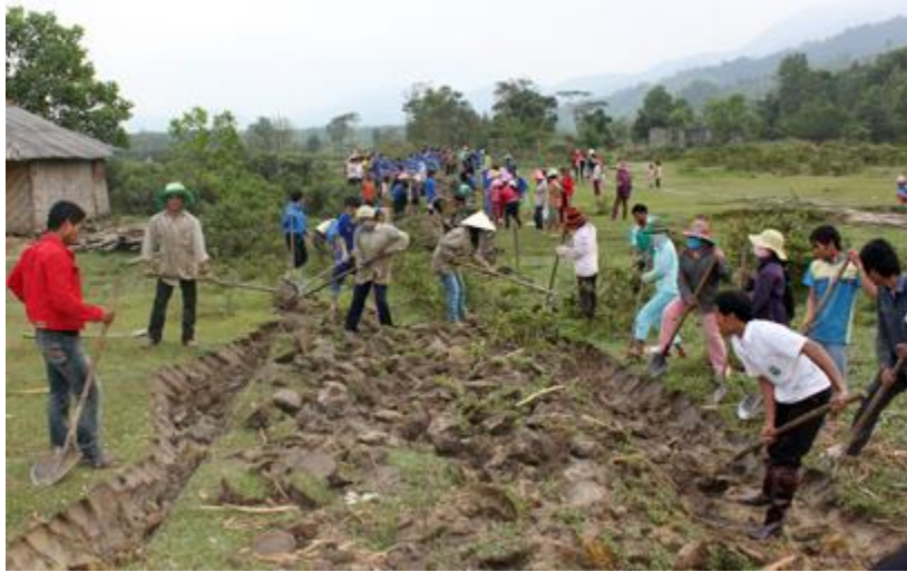
DTU students rebuild a small road leading to Mr. Le Ninh Tuoi's house
